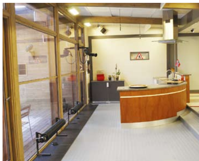
Installed by a window the ribbed pipe radiators effectively counteract cold draughts that frequently form by large glazed areas.
